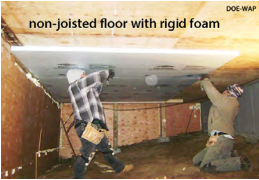
Non-joisted floors with rigid foam: Workers fasten rigid foam to a non-joisted floor with plastic-cap nails.
