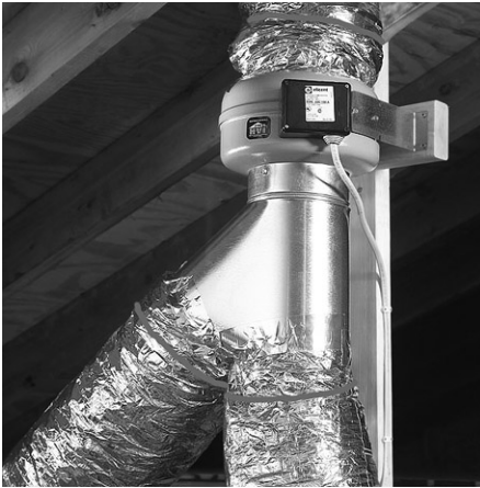
In-line fan in attic: A Y exhausts airflow from two bathrooms for both local exhaust and whole-building ventilation.
