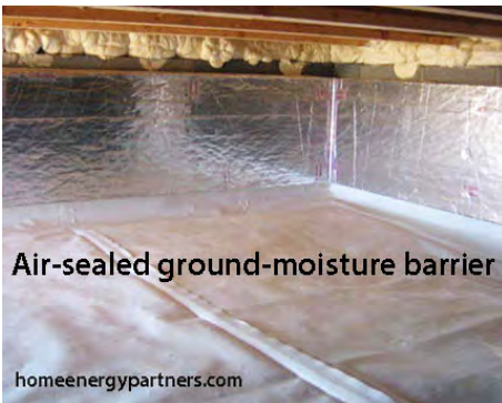
Ground-moisture barrier: An airtight ground-moisture barrier blocks water vapor and gases coming up from the ground.
